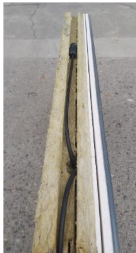
Figure 5.18: Demo-site 4, Groove created on the top horizontal edge to provide cable passage
