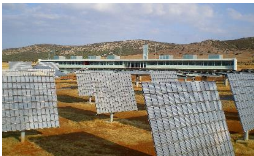
Figure 2.2: ISFOC 800kW CPV power plant
