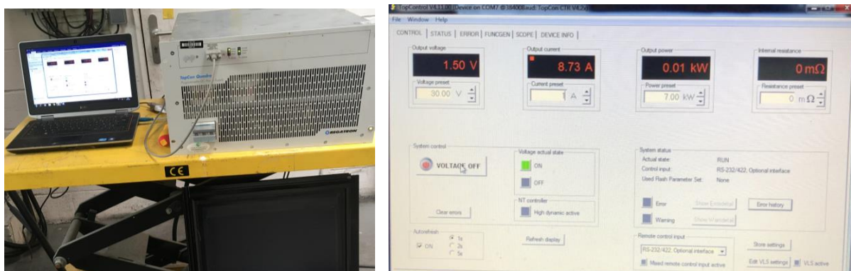
Figure 26. DC PV GENERATOR (10 kW DC) – SBI preliminary settings before mockup connection Load device and remote control to test load on CIGS module (left) / User interface with load level (right) – Same procedure is used for crystalline modules
