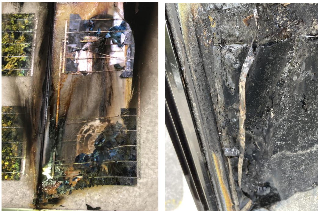
Figure 31. Busbar status after fire test, continuity test are performed, and module are still working / glass-glass module on veture kit cladding (Left) – thin film module polymeric-based on veture kit cladding (Right)
